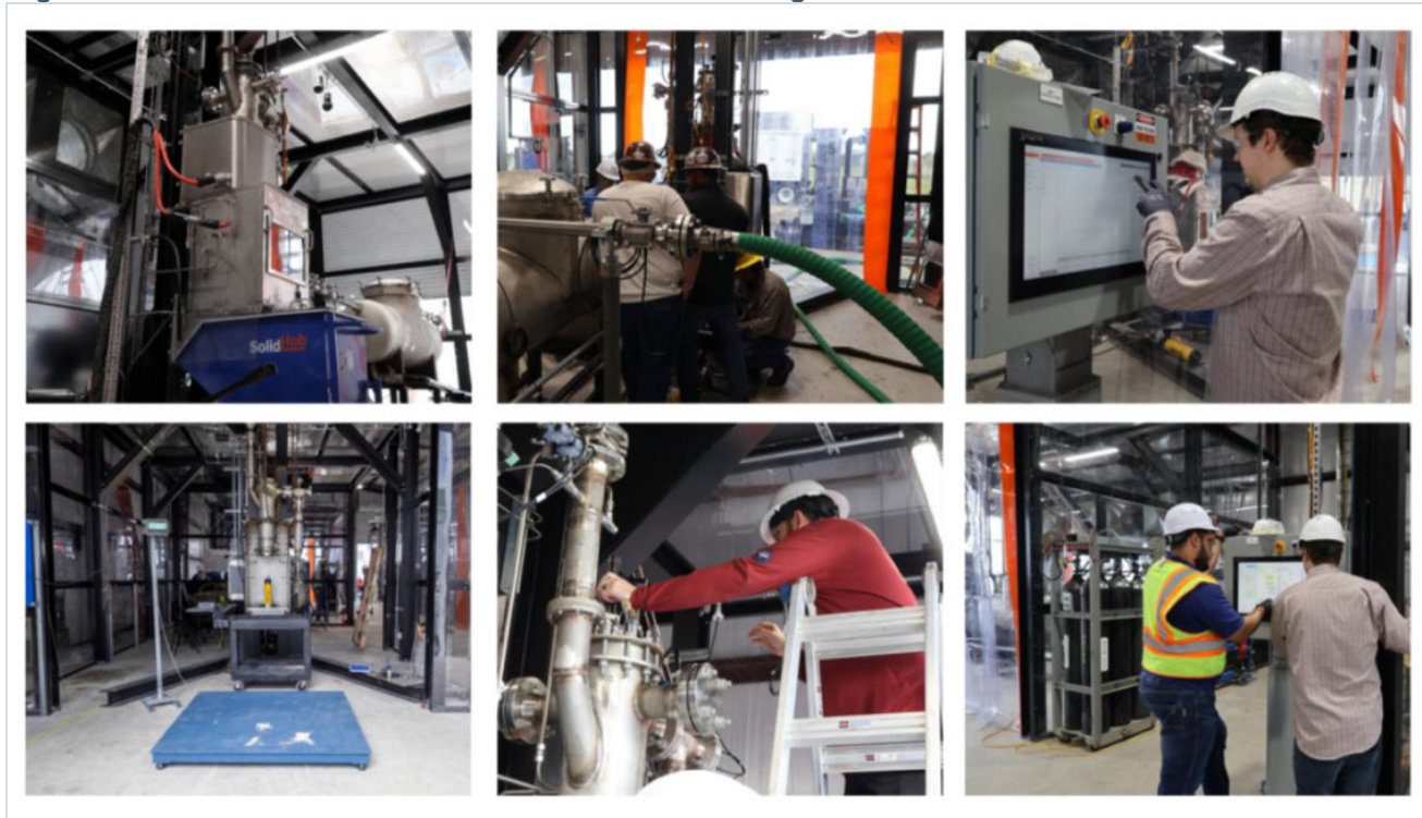
Figure 15: Metallium's small modular reactor commissioning
